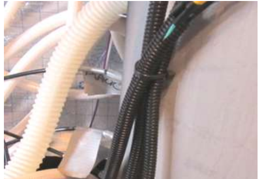
Fig. 19 A IP 66 wire pairs and 12V supply wires sheathed over and tie wrapped
