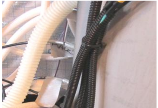
Fig. 18 A IP 66 wire pairs and 12V supply wires sheathed over and tie wrapped
